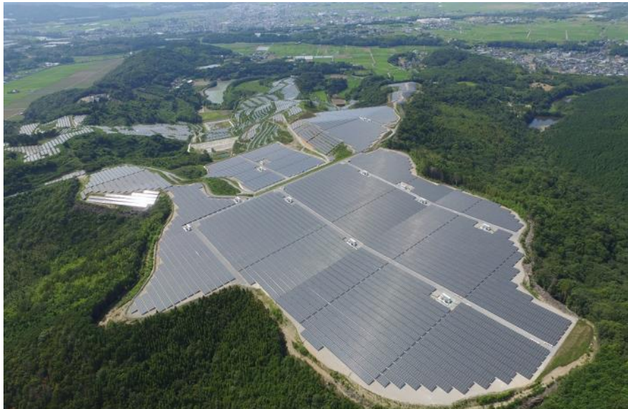
Civil engineering land development for SGET Usa Mega Solar Power Station (Hitachi Ltd.)
